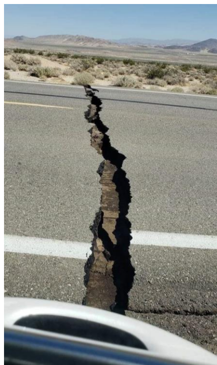
Figure 1. Trona Rd after the Earthquake near Ridgecrest, CA today. (San Bernardino County VOAD)
