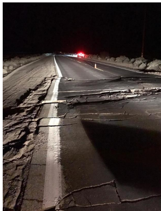
Figure 2. California State Route 178 southwest of Trona after the July 5, 2019, magnitude 7.1 quake. (U.S. Geological Survey)
