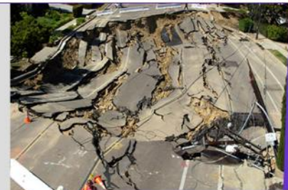
Photo Credit: Michael Hart La Jolla Landslide Headscarp
