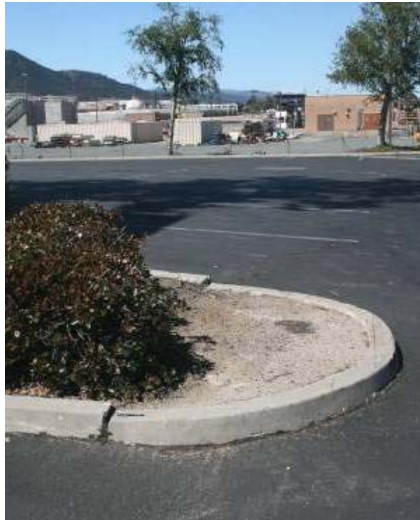
Broken curbs vicinity of Murrieta Creek fault zone in Temecula
