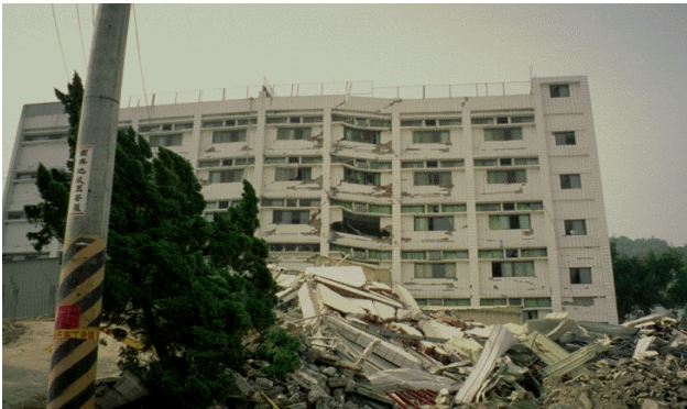
Figure 19 The primary trace of the Chelungpu fault passed beneath this apartment building in Wu Feng, producing about 2 m of vertical displacement through the building (Photo by K. Kelson).
