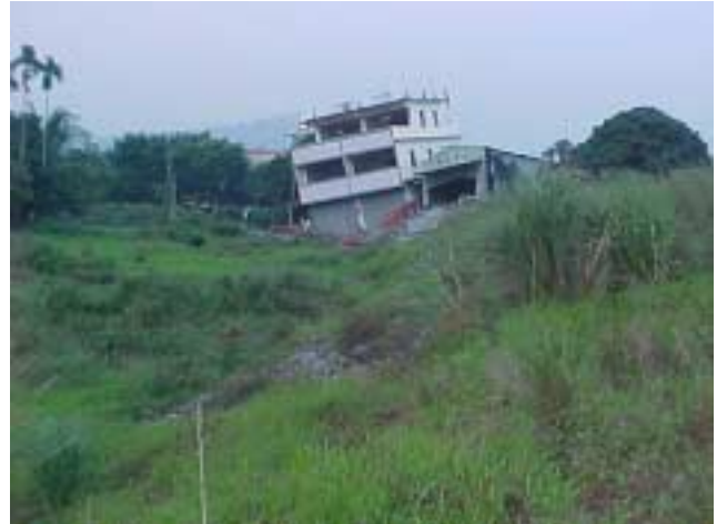
Figure 20 North-facing subsidiary fault in hanging-wall block and local ground deformation damages this house and warehouse. This site is located southeast of Shihkang Dam and south of the primary fault ruptures running along the Tachia River in this area (Photo by J. Bray).
