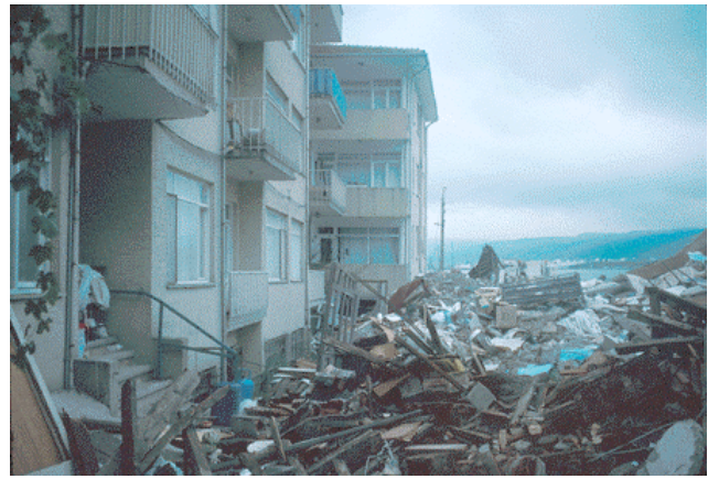
Figure 7 Apartment house shown on right side of photo, which collapsed due to surface rupture. Fault passes across the middle of the photo between the two standing apartment houses; the far apartment house has been offset about 3 m from its original alignment with the near apartment house (Photo by F. A. Swan from Lettis et al. 2000).
