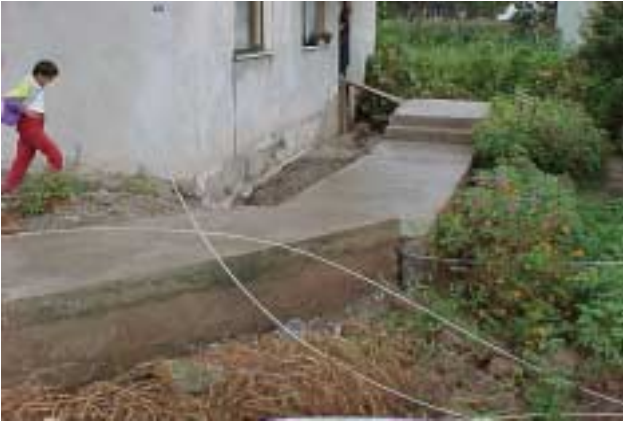
Figure 13 Well-built 2-story house in Arifiye is not damaged although the primary surface fault scarp passed beneath it with over 3 m of right-lateral displacement. In response to the underlying fault movement, the stairs leading to the house have been offset relative to the house (Photo by J.D. Bray).
