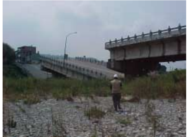
Figure 17 Collapse of bridge directly east of Shihkang Dam due to tectonic compression (Photo by J.D. Bray).
