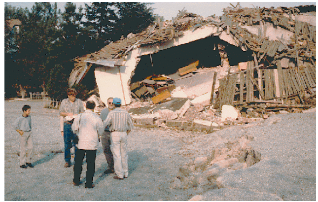
Figure 11 Fault rupture destroyed a primary school building in Kullar (Photo by L.S. Cluff; from Lettis et al. 2000).
