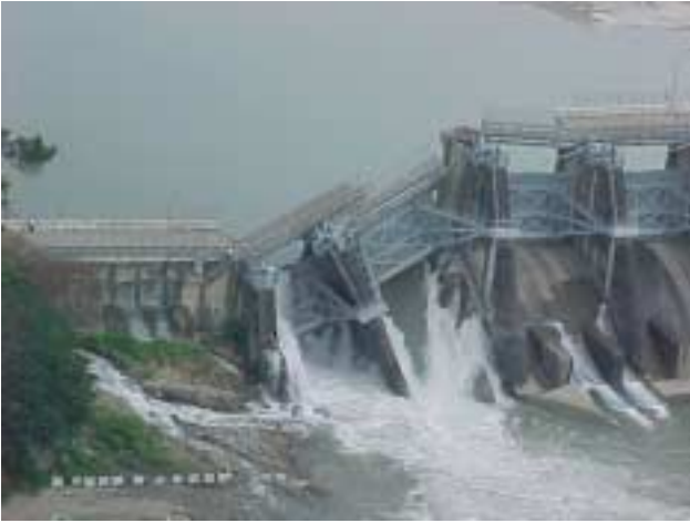
Figure 15 View to the east of surface fault rupture through Shihkang Dam (Photo by J.D. Bray).
