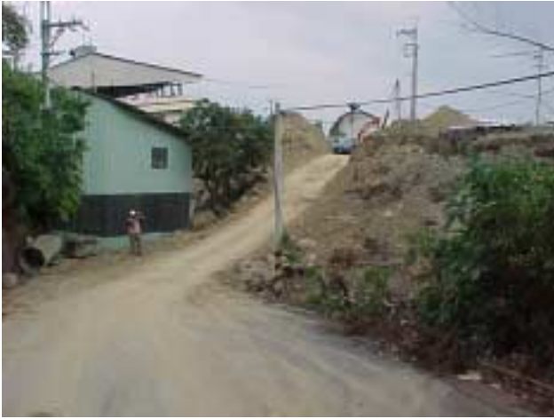
Figure 18 Fault scarp that is about 5 m high passes close to, but does not damage, a simple steel-framed warehouse that is located on footwall side of shallow thrust fault (Photo by J. Bray).
