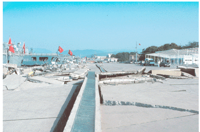
Figure 9 Fault offset of about 2 m heavily damaged this dock at the Gölcük Naval Base, which was fixed to the ground with piling (Photo by F.A. Swan; from Lettis et al. 2000).
